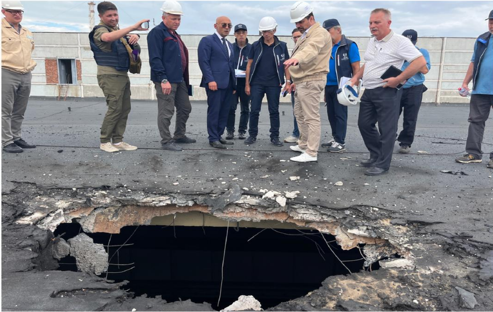
The IAEA team observes the damage caused by shelling on the roof of the special building at the ZNPP that houses, among other items, the fresh nuclear fuel and the solid radioactive waste storage facility. (Photo: IAEA)
