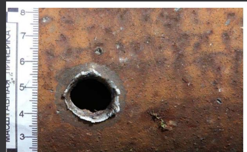
Damage to metal that was reportedly caused by shrapnel, observed by ISAMISU at the location where the intercepted drone had allegedly fallen on the night of 24–25 September 2025. (Photo: SUNPP)
