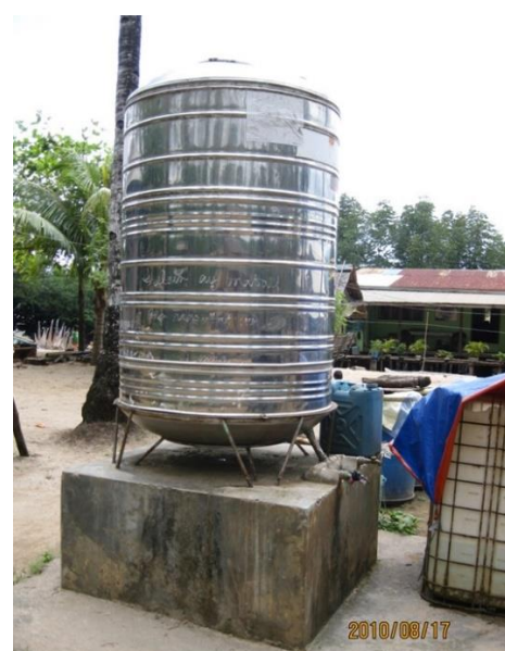
Figure 5: Delivery water tank
