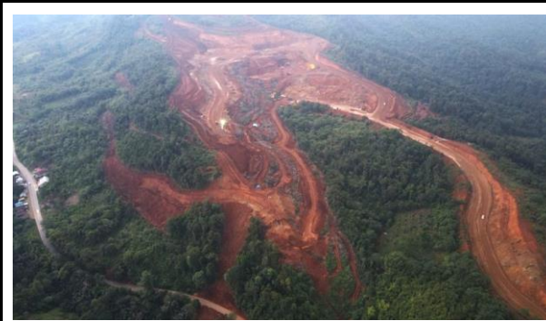
PTVI's mining operation expanded into the area right above the community water source and their residential houses in Asuli village. (Photo: July 2022)
