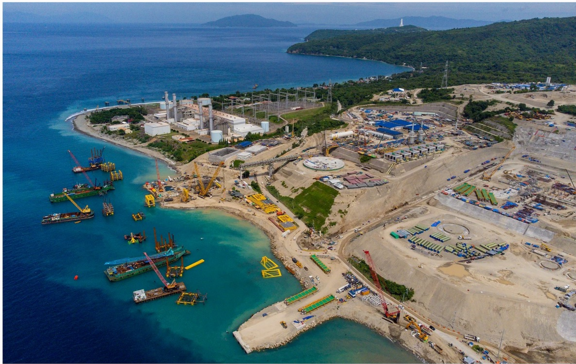
Look: Drone photos much development has already occurred in the projects' site as of August 2022. DAR confirms that this was done by SMC-EERI and Linseed-AG&P without proper land conversion applications or permits. Photo by B. Sepe.
